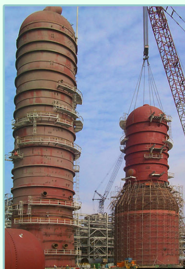
▲C210 汽油分餾塔 Gasoline Fractionator SA516-70 \phi 12.2 m x 67.9 m L x 1,092 Ton
