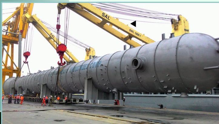
▲C-1401 乙烯分餾塔 Ethylene Fractionator SA516-70 \phi 6.7 m x 92.7 m L x 762 Ton
